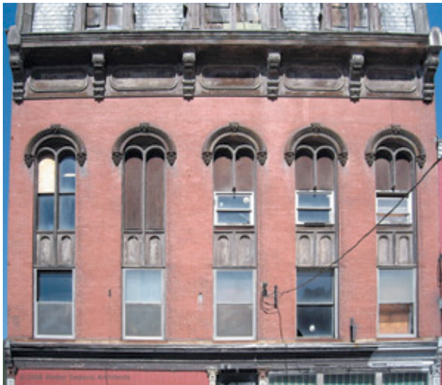
The damage wrought by replacement windows is self-evident and increasingly pervasive. All photos: © Walter Sedovic Associates
